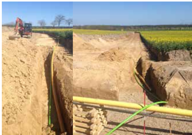
Avacon, biogasleiding, 16 bar
