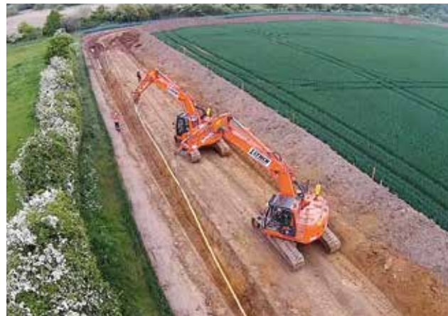
Fakenham, Feed-in biogasleiding, 19 bar
